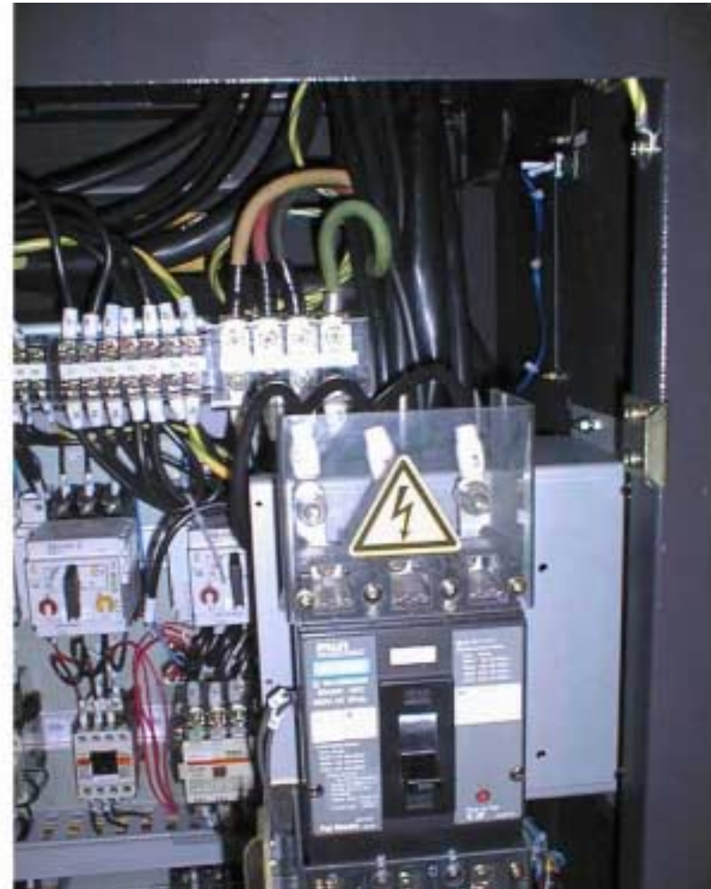
Coma 567 main power connection inside of electrical enclosure
