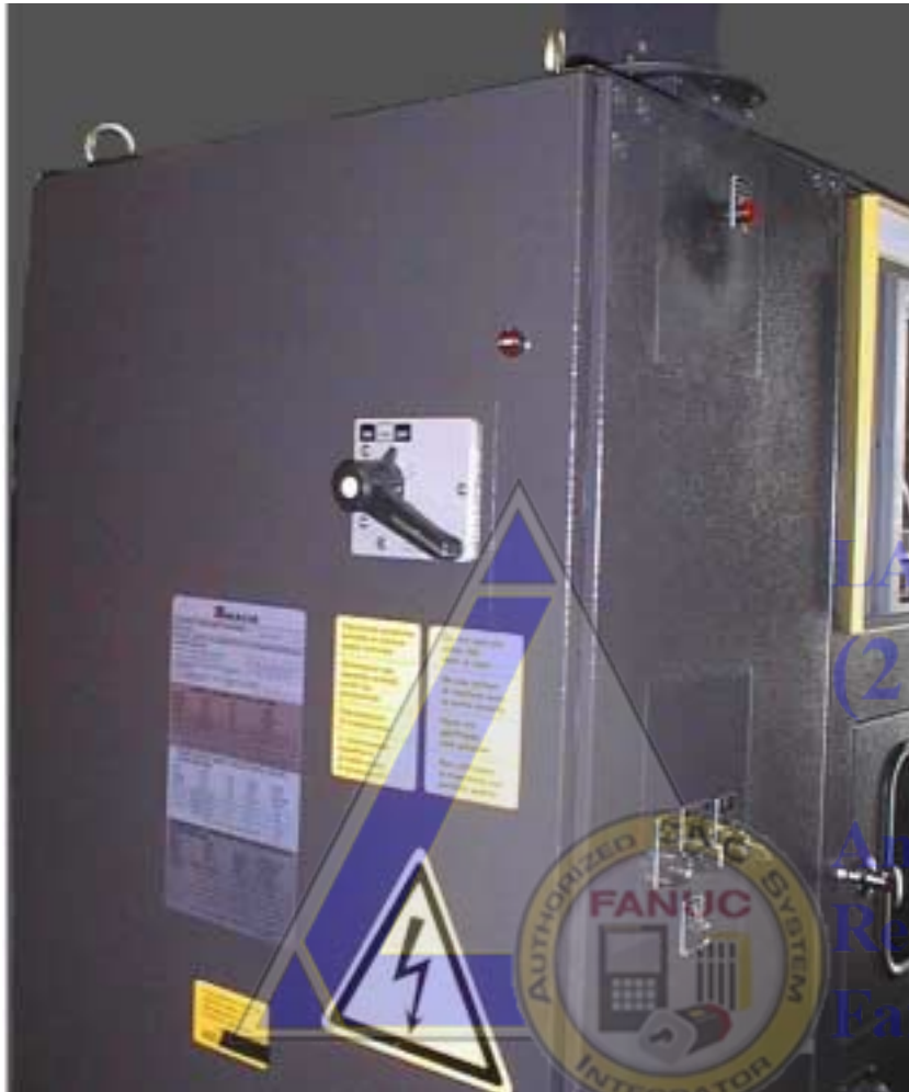
Coma 567 left side of electrical enclosure
