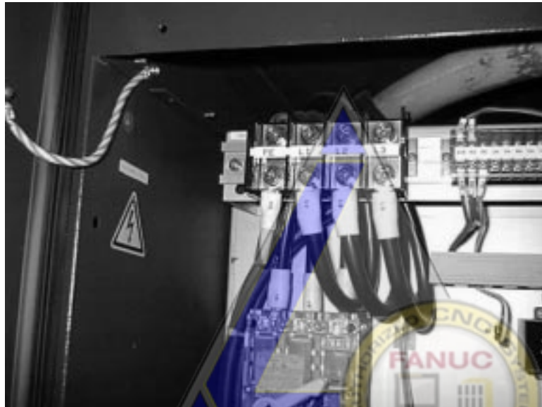
Vipros electrical enclosure
